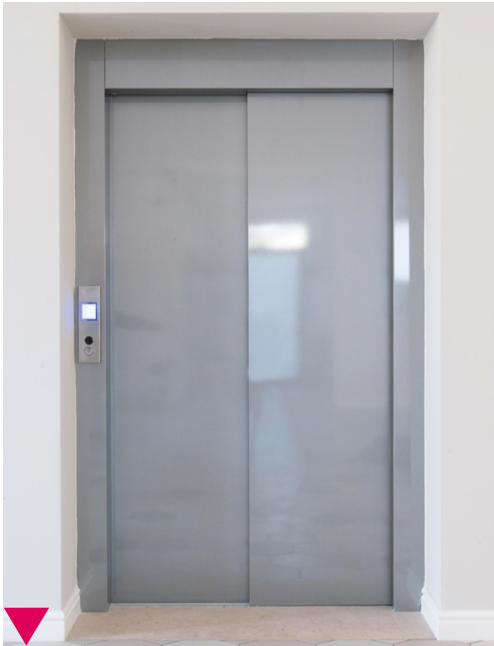
EXAMPLE OF A SKINPLATED AUTOMATIC DOOR
